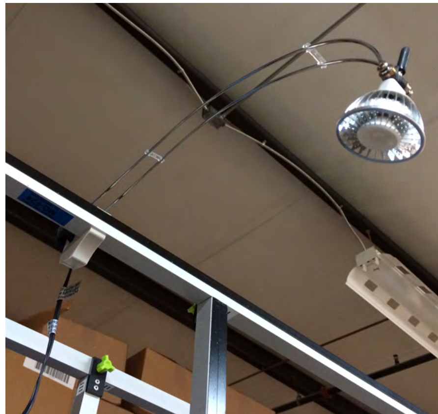
WAVE STEM LIGHT (INSTALLED)
