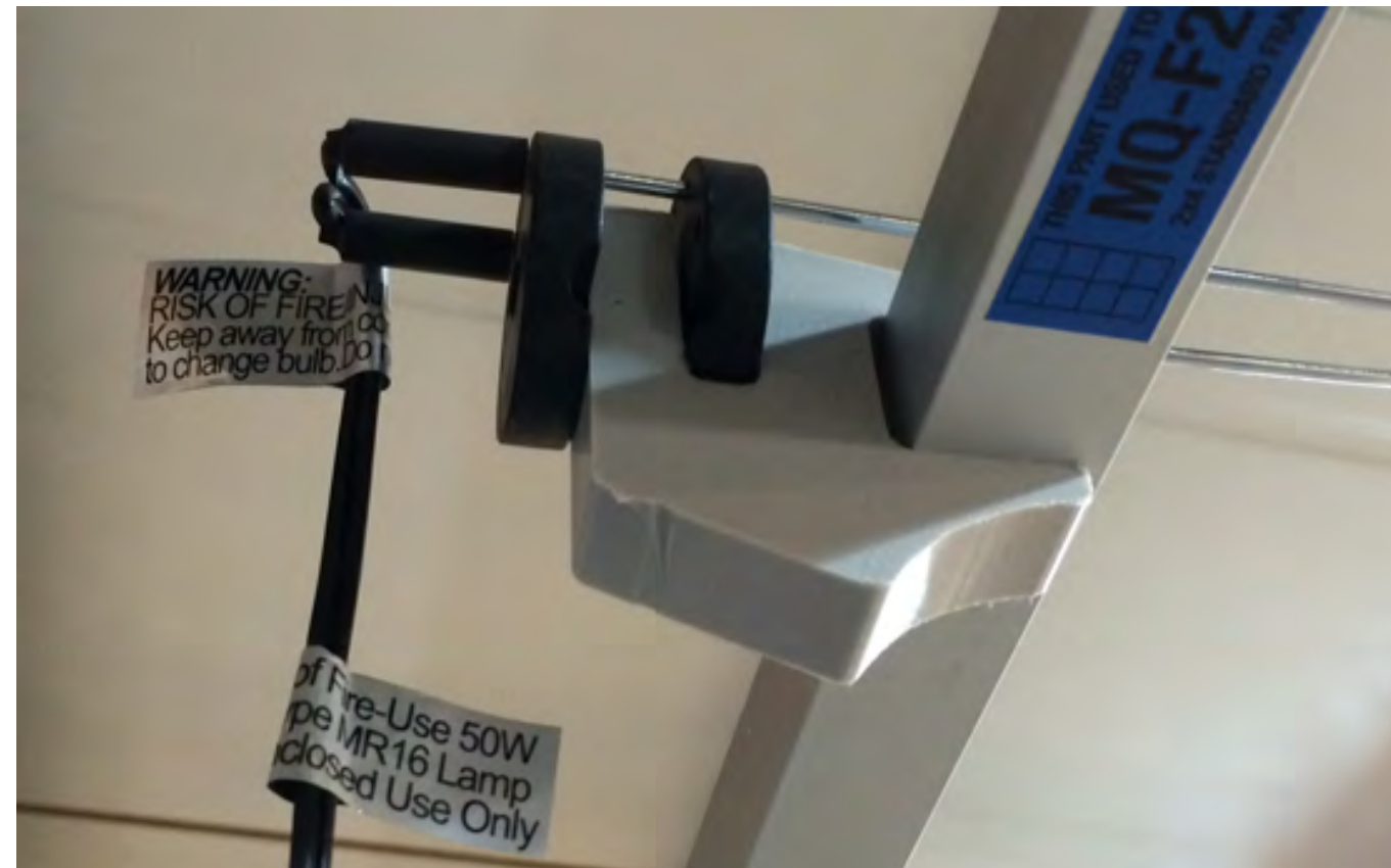
WAVE STEM LIGHT (INSTALLED - CLOSE UP)
