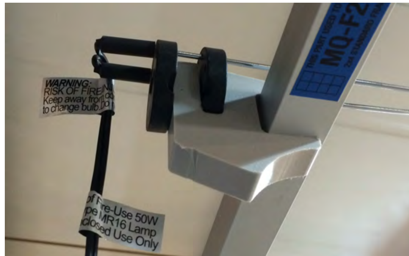
WAVE STEM LIGHT (INSTALLED - CLOSE UP)
