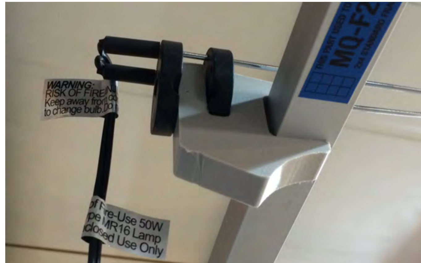
WAVE STEM LIGHT (INSTALLED - CLOSE UP)
