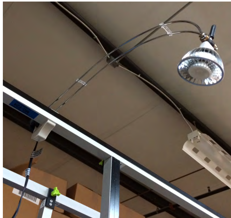
WAVE STEM LIGHT (INSTALLED)
